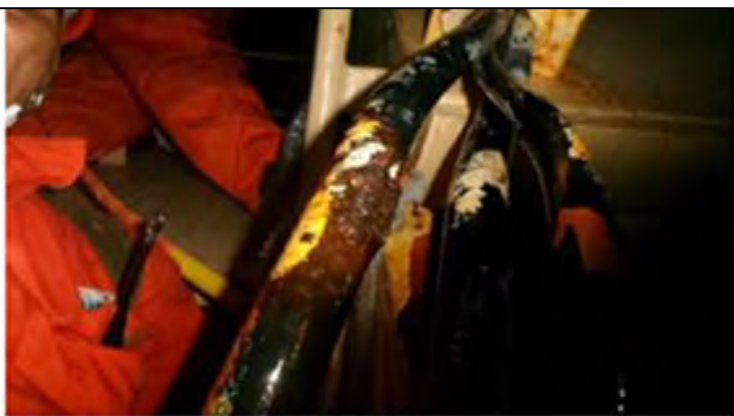
Part of the hose burst
